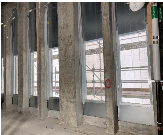
Pictured: Windows in the process of being reinstalled in the Hepburn Tower.
