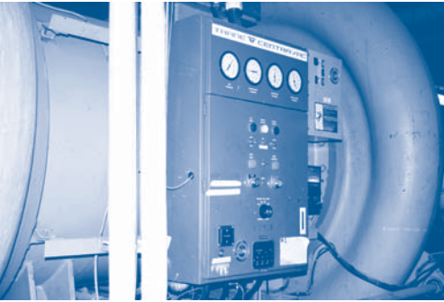
Chiller Control Unit, Queen's Park Complex
