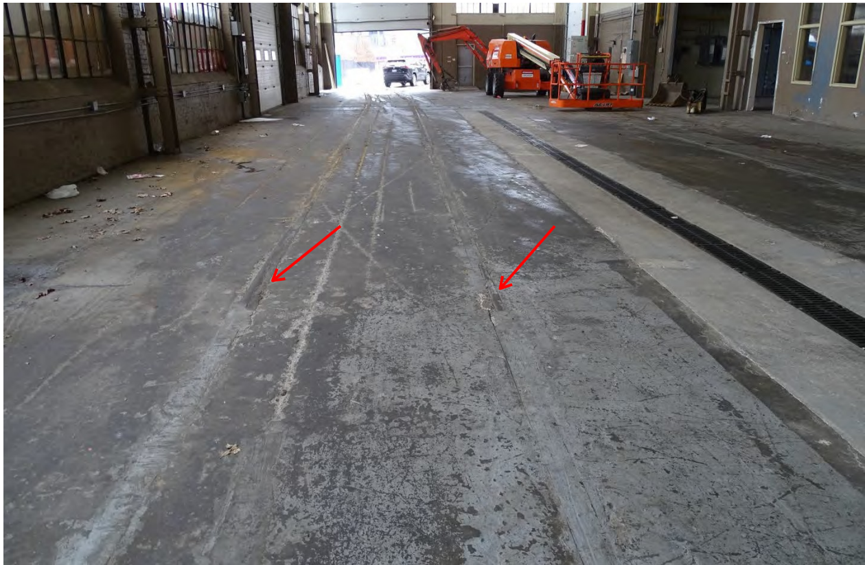
Figure 77: 1935 Machine Shop showing railway tracks embedded in the slab Credit: SBA, February 2021
