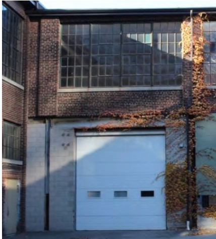
Figure 63: 185 Eastern Avenue – 1935 Machine Shop Post 1940s Addition – East Elevation Credit: SBA, November 2020
