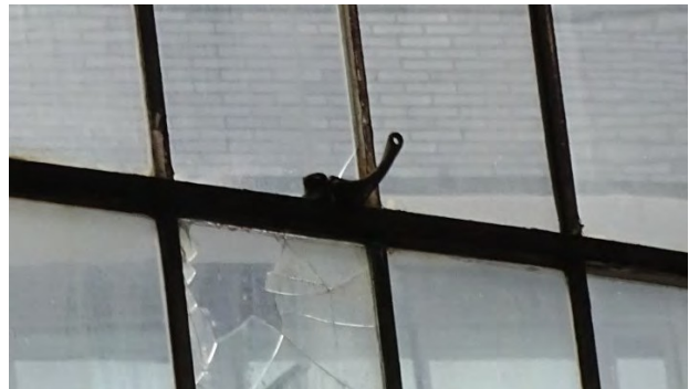
Figure 70: Original window hardware Credit: SBA, February 2012
