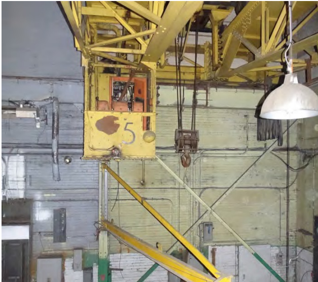
Figure 28: Gantry Crane at Northwest Corner Credit: SBA, November 2020
