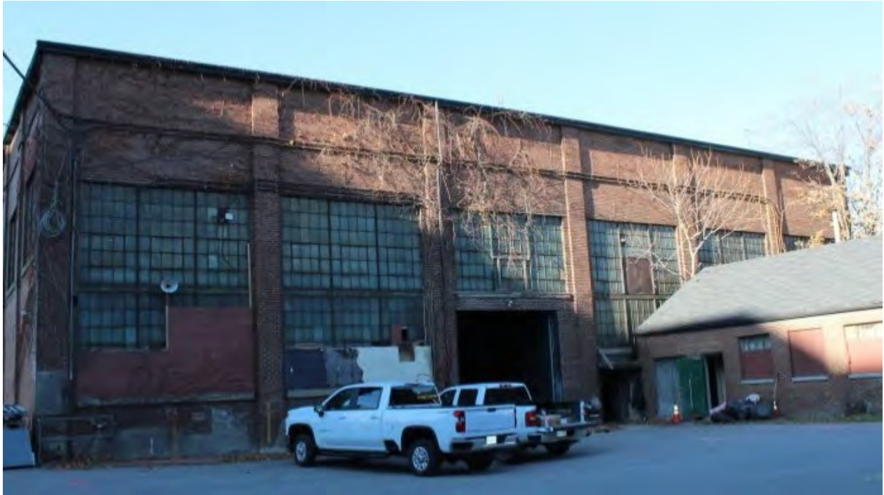
Figure 20 East (Side) Elevation, Looking Northwest: Prior to Partial Demolition Credit: SBA, November 2020
