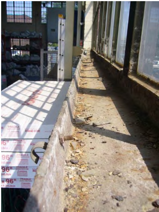
Figure 69: C channel of south wall of the original shop rotating outward. Credit: Commonwealth, 2008
